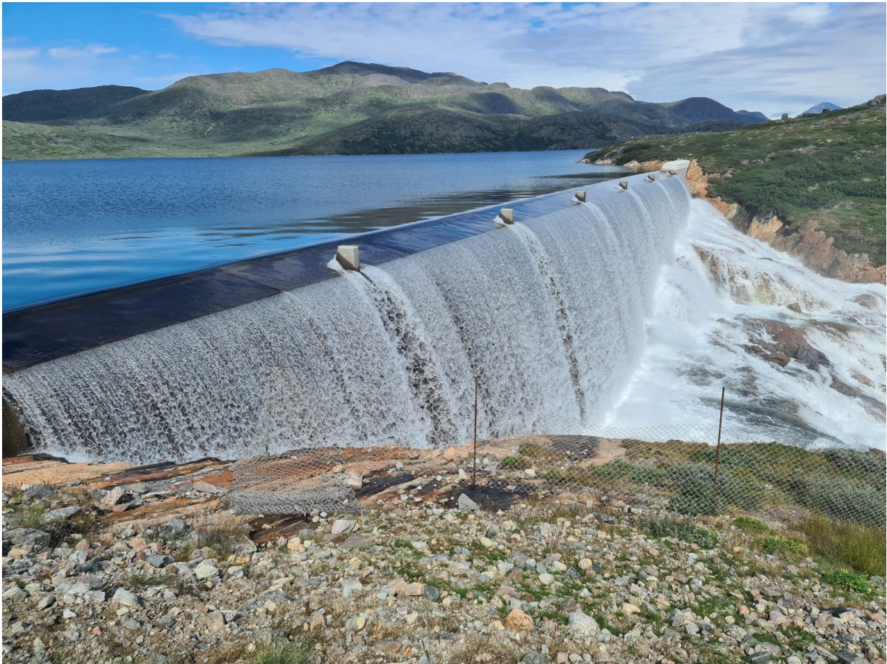
Dam of a small-scale hydropower station of 7MW in the South of Greenland, credit: Claus Andersen-Aagaard.
