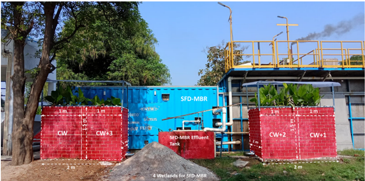
SFD-MBR and Constructed Wetlands + pilots being demonstrated at Jajmau STP, Kanpur
